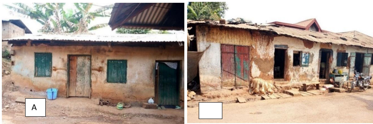
Plate 2A: Single room housing in need of major repairs in Old Town B: Dilapidated housing quality in Old Town Source: Field work, 2019
