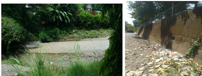
Fig 3. The condition of the river Bajak
