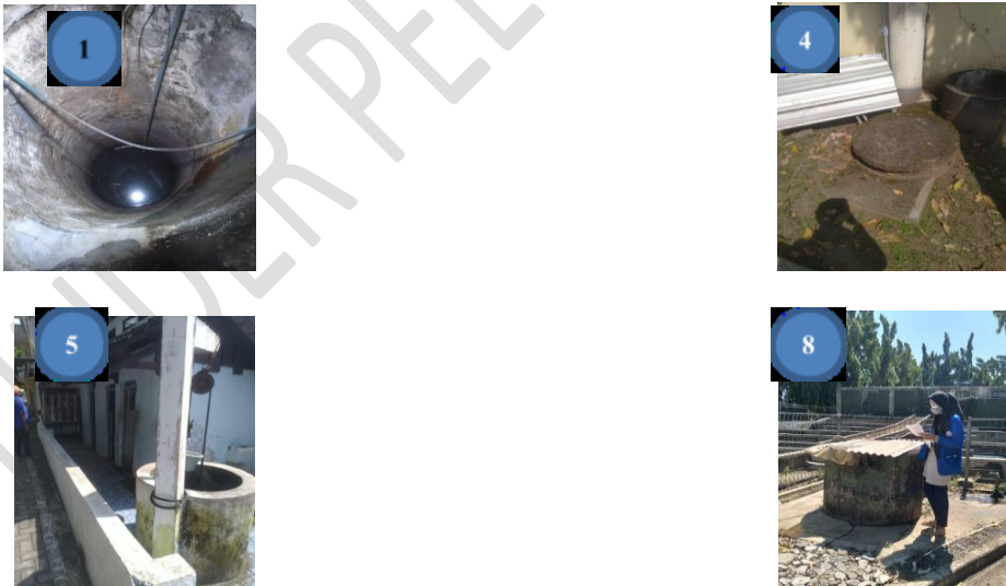
Fig 4. . The community well conditions
