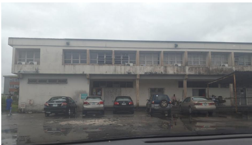
239 240 Plate 2: Dampness of walls 241
