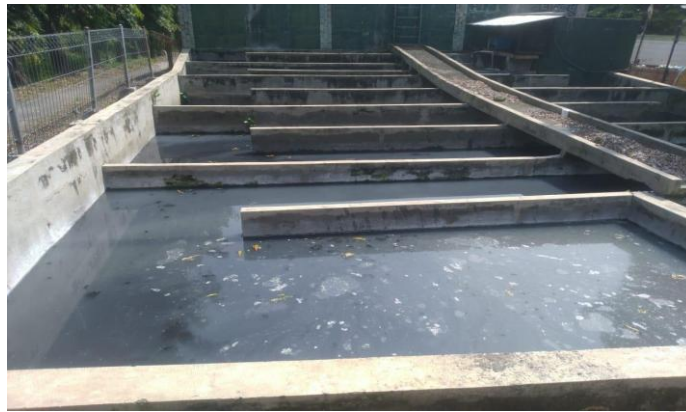
Fig 3. Tofu Waste Treatment Plant, Central Lamper Village, Semarang-Indonesia
