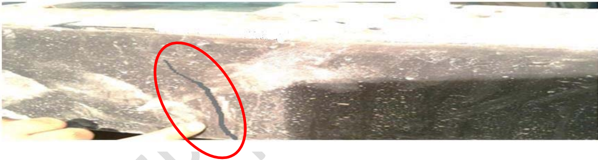
Fig.10. Failure mode of sleeper S 10 under static load on rail seat section
